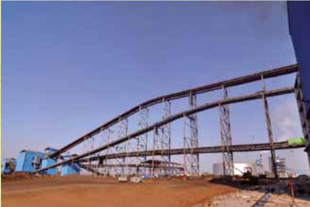
Bagasse and Coal handling system
