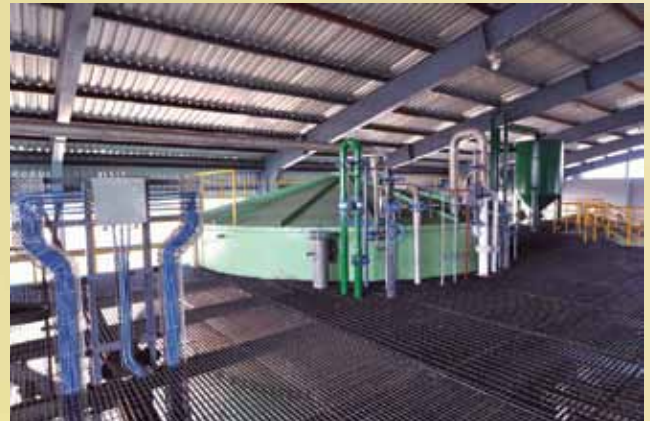
Fermentation Section of Distillery Plant
